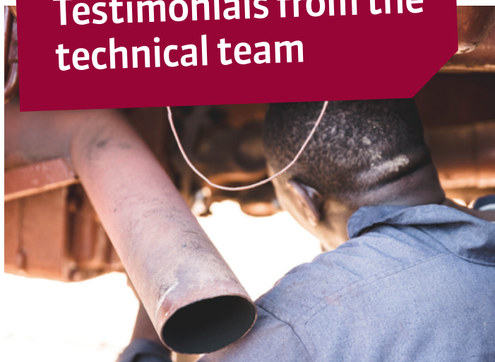
God made possible the repair of the truck and a scheduled start
