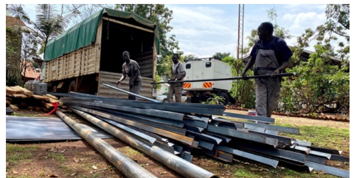
All material for the construction for the fence, toilets, cesspit and guest house were purchased in Kenya then transported by truck for three days to South Sudan.
